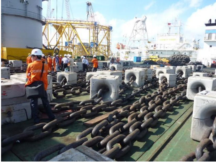
9 lengths of RQ4/RQ3 mooring chain lying on the Truong Sa Crane barge prior to offshore installation.
