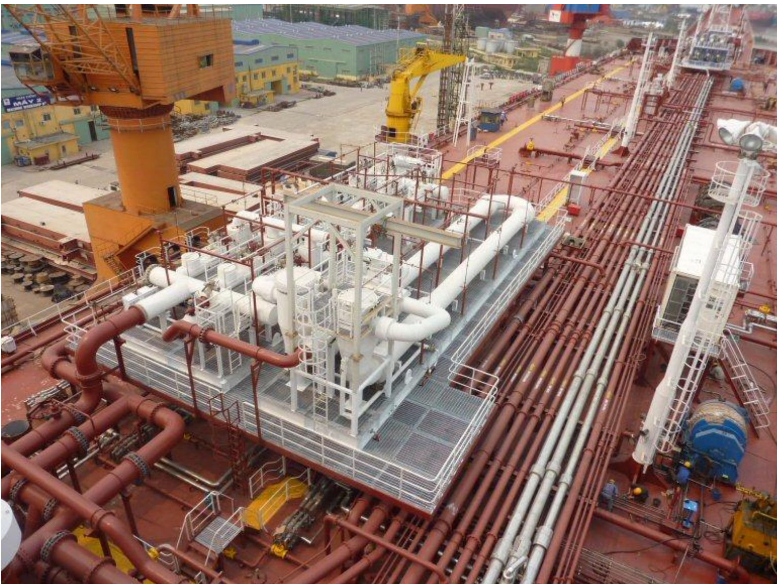
Metering unit installed on deck
